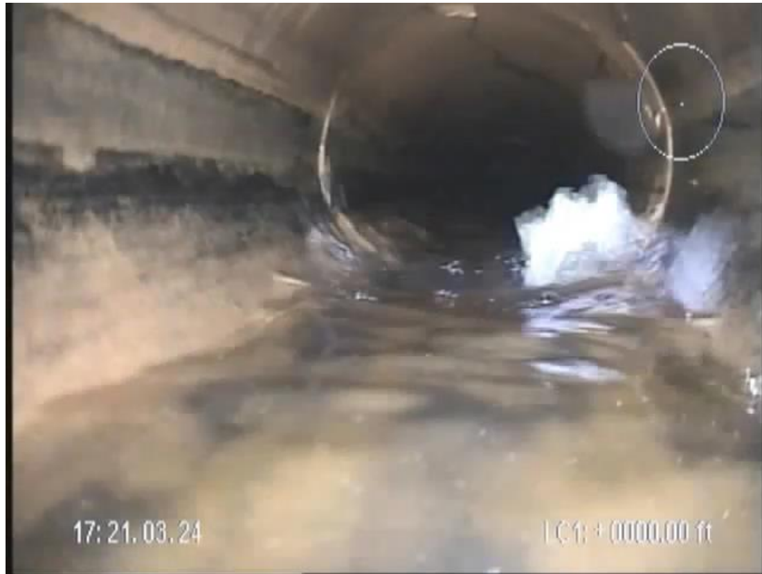
IGJ (Infiltration Gusher Joint) – separated joint
