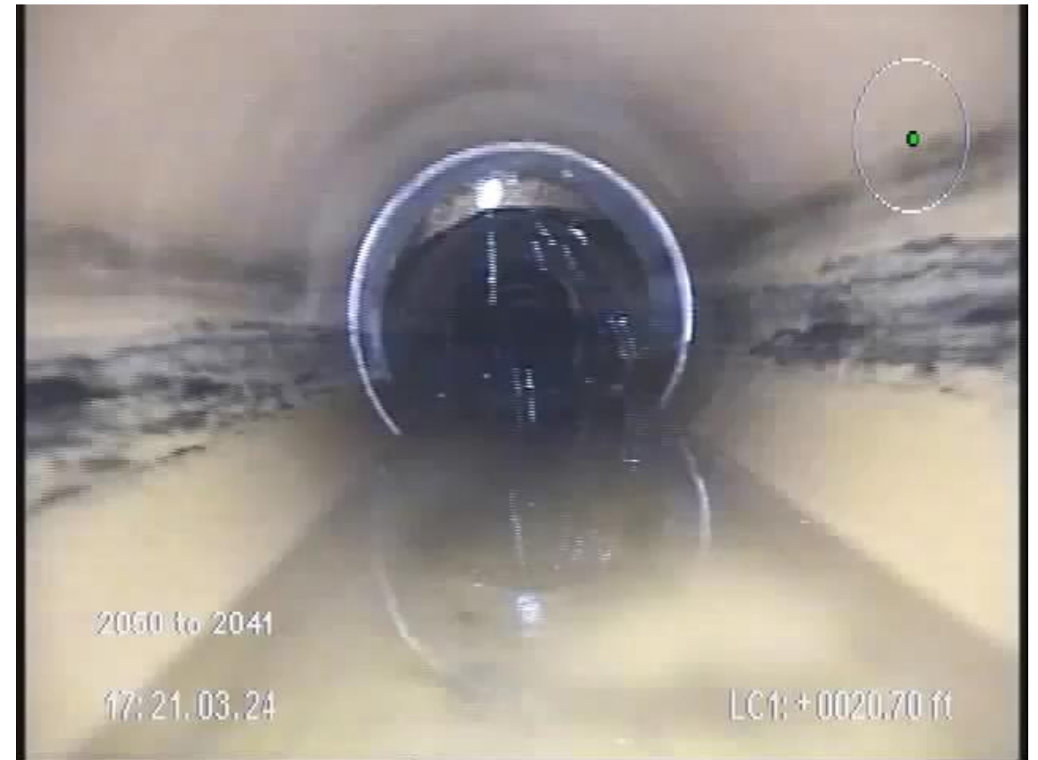
IRC (infiltration runner connection) due to a defective connection/tap
