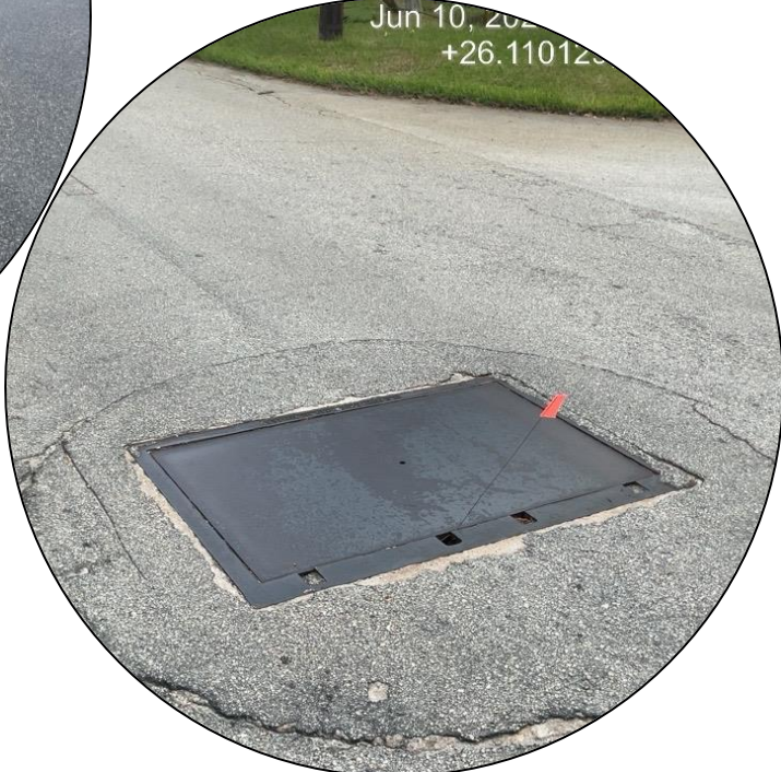
Pump Station Defects
