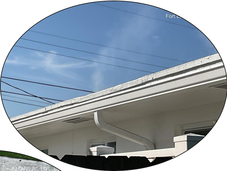
Stormwater Cross Connections
