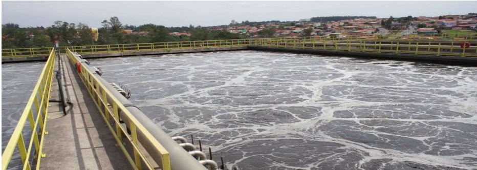
Traditional Wastewater Aeration
